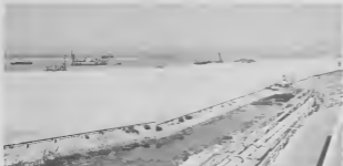
Dredge "George", working for Nederlands Harbour Works, began dredging and land reclamation work on April 2, 1969.
